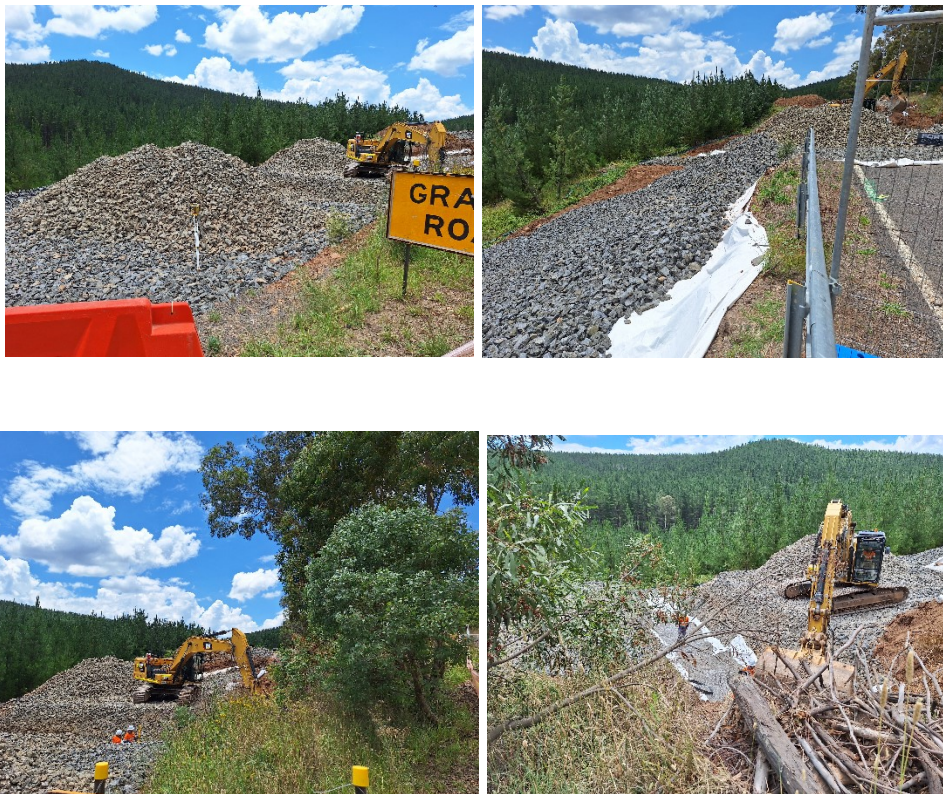
Four Mile Creek Road - Landslip
