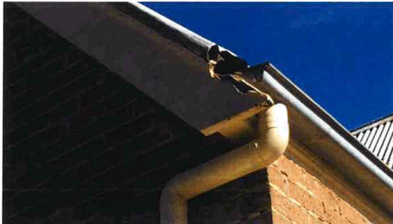
Figure 26 Missing spear point and flashing and eroded barge board end. The quad gutters have decayed and should be replaced with galvanised ogee guttering
