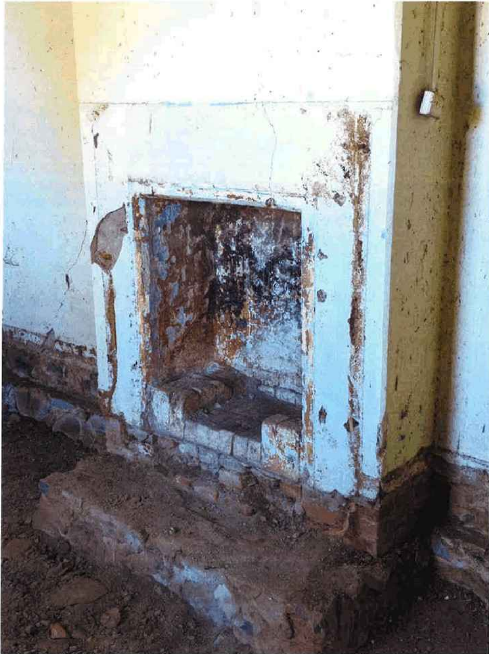
Typical chimney noting the brick construction and tied in nature of the cross walls. No more excavation should be undertaken so as not to undermine the foundation.
