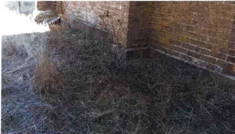
Figure 9 Typical view of the perimeter where weed growth is against the building promoting rising salt damp
