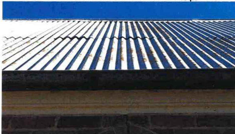
Figure 15 While the roof sheeting looks fine, many fixings are raised and the end laps have opened allowing wind blown rain to enter the roof space.
