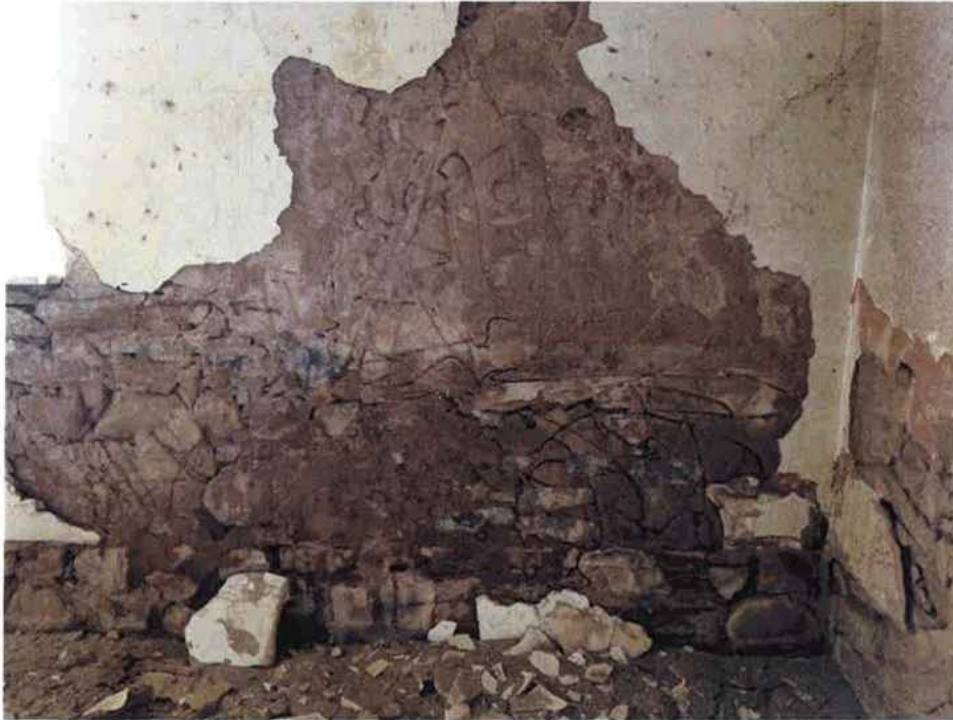
Removing the drummy render is essential in restoring the cracks and then re-plastering.
