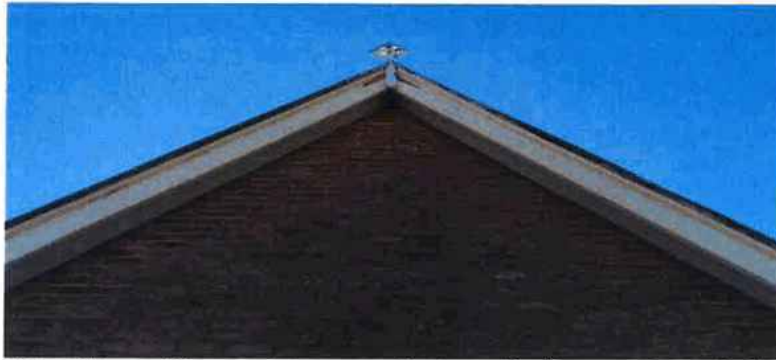
Figure 18 The remaining cross in place. Replicas can be made from this one.
