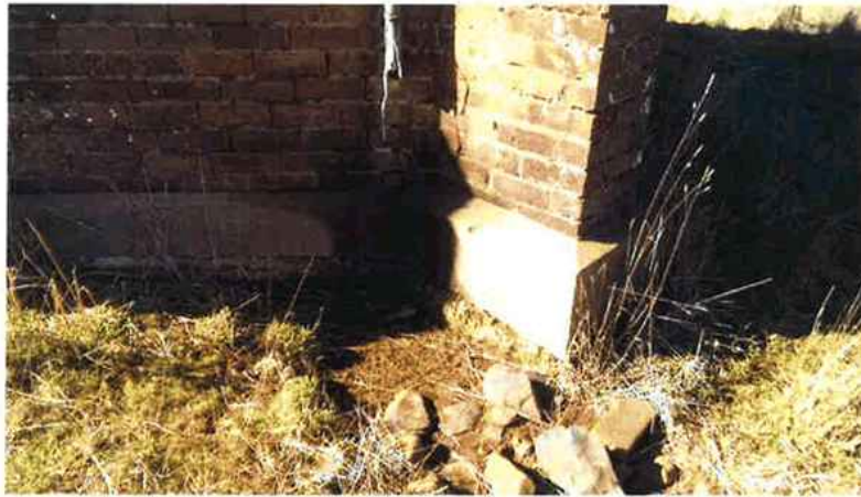
Figure 20 Water damage and missing downpipe
