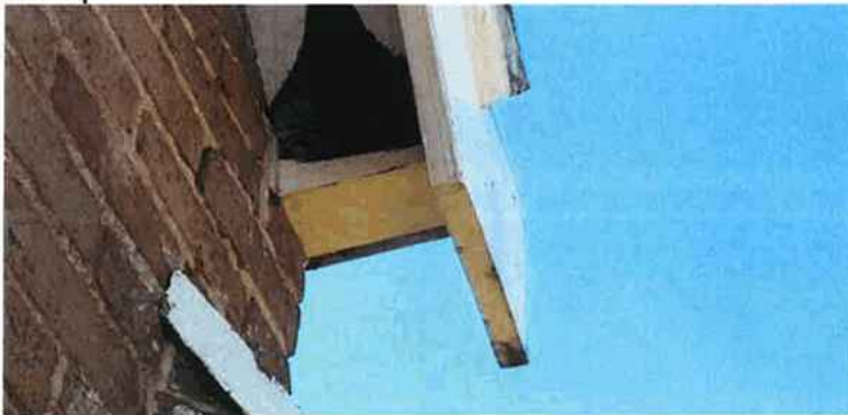
Figure 17 Damaged timber at the eave and barge board junction
