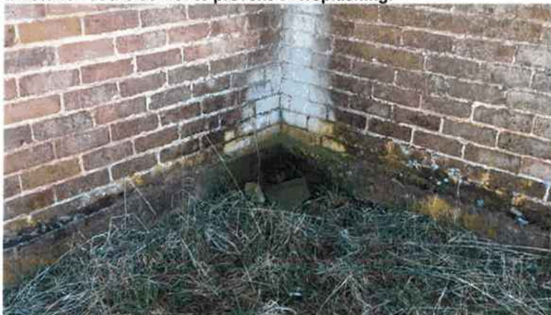
Figure 13 The solution is an extra downpipe in this area with the water carried 4m clear.
