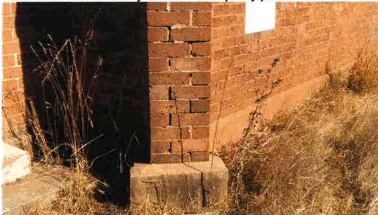
Figure 25 Missing pointing on the exposed piers
