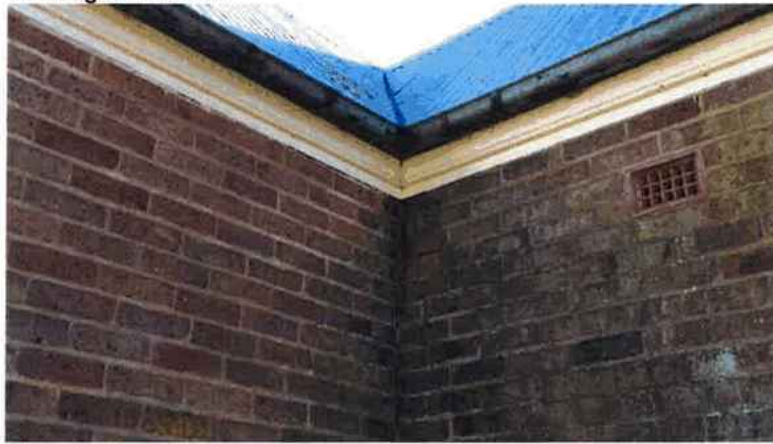
Figure 12 The internal corner is not draining to the downpipe and overflows are damaging the brickwork and foundation. Refer the following image. Install an acroterion at the corner to prevent oversplashing.
