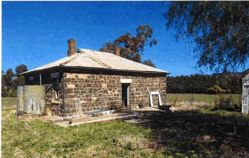
View of the rear of the cottage noting the hipped roof form with gable vents and pair of brick chimneys – critical in the stability of the building
