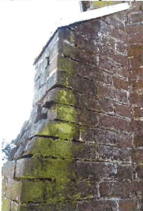
Figure 19 Water damage requiring brick repair and replacement
