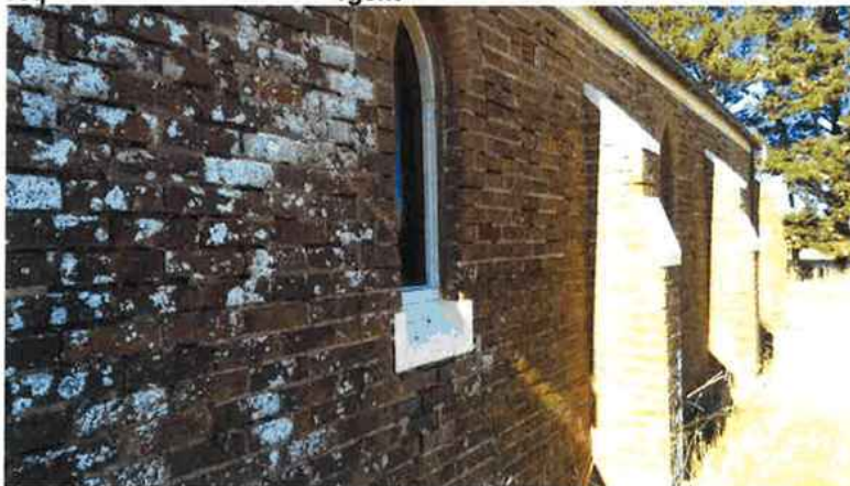
Figure 22 Side elevation showing the missing pointing caused by the leaking guttering. Simple bristle brush or mild pressure washing to the brick walls being careful not to remove friable materials in the walls and windows.
