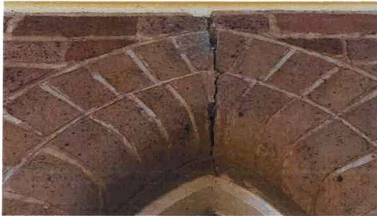
Figure 14 General foundation movement leads to shrinkage and expansion/heave cracking. The initial solution is a 1200mm wide gravel perimeter apron. After a minimum of 6 months the movement cracks could be re-pointed.
