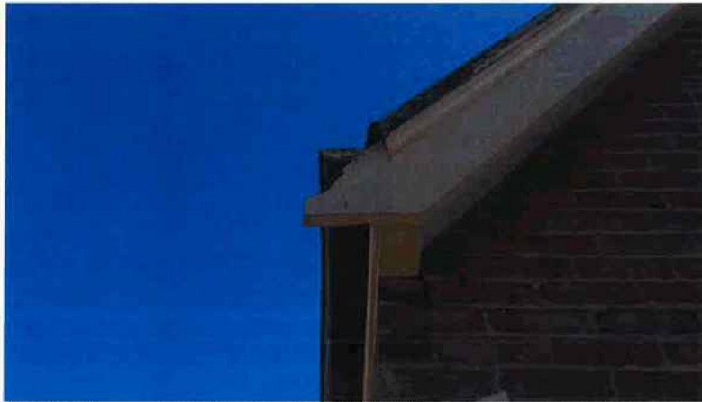
Figure 11 A missing barge roll flashing has allowed water to run off and damage the barge board end
