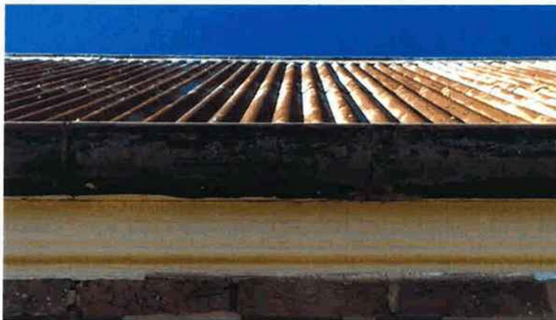
Figure 21 Note rust damage and raised fixings. The guttering is completely eroded through and replacement galvanised steel guttering and downpipes are required. This is the most urgent task.
