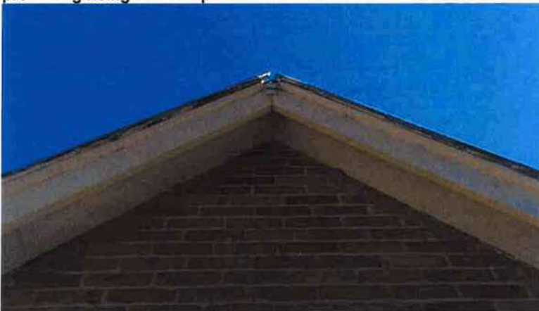
Figure 10 The missing cross leaves the two barge roll flashings open and water can affect the roof and barge boards
