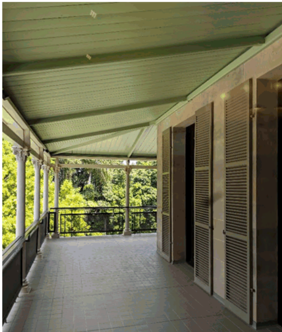
Photo 3 This same verandah also shows the balustrade and the traditional green colour used for verandah timbers and linings.
