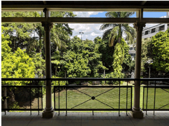
Photo 2 The balustrade is fine perforated wire in painted steel frame fixed to four rods which span between the floor and handrail.
