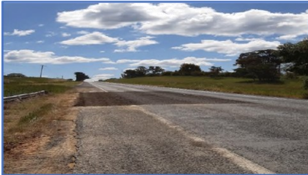
Heavy patching – MR61 Escort Way
