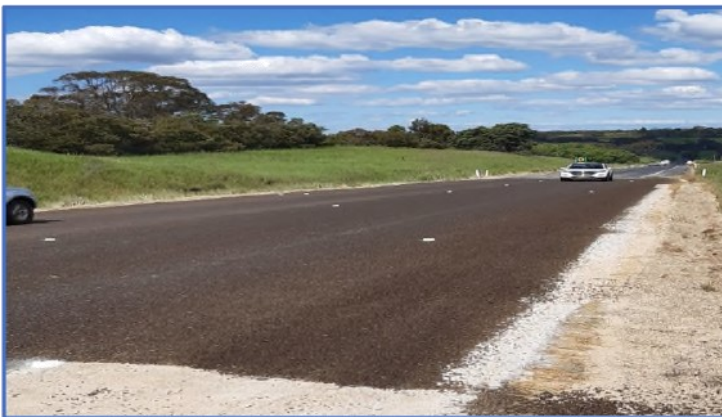
Heavy patching – MR61 Escort Way
