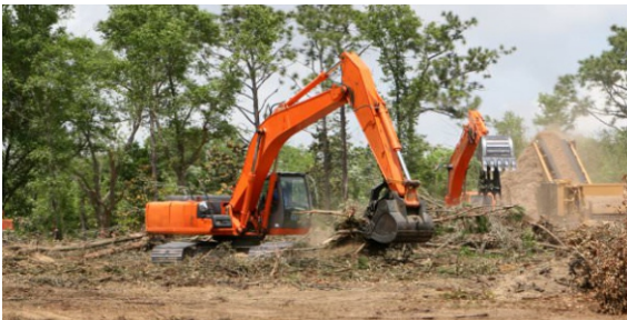
The site is cleared; removing all vegetation and a large amount of soil.
