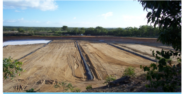
A network of gravel and pipes are constructed at the bottom of the landfill cell to capture and remove the polluting leachate and store the liquid in ponds for treatment.
