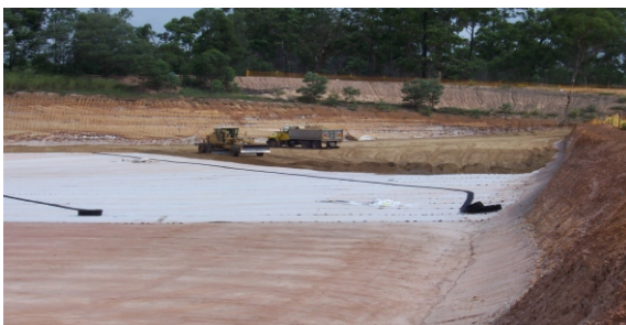
A waterproof membrane is then placed over the exposed soil to prevent leachate from soaking into the surrounding soil and groundwater. Material such as clay is spread across the membrane to form another protective layer.
