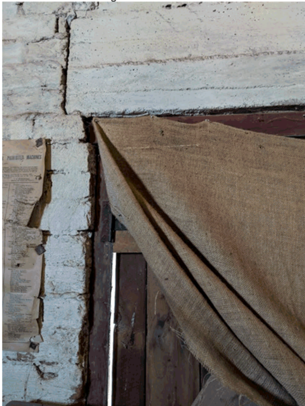
A Detail view of the movement cracks in the lintel
