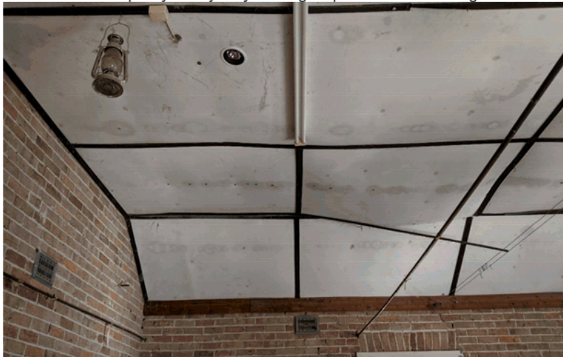
Figure 2 The images indicate that the ceiling is not sound, replacement with new plasterboard and battens will lessen the load considerably
