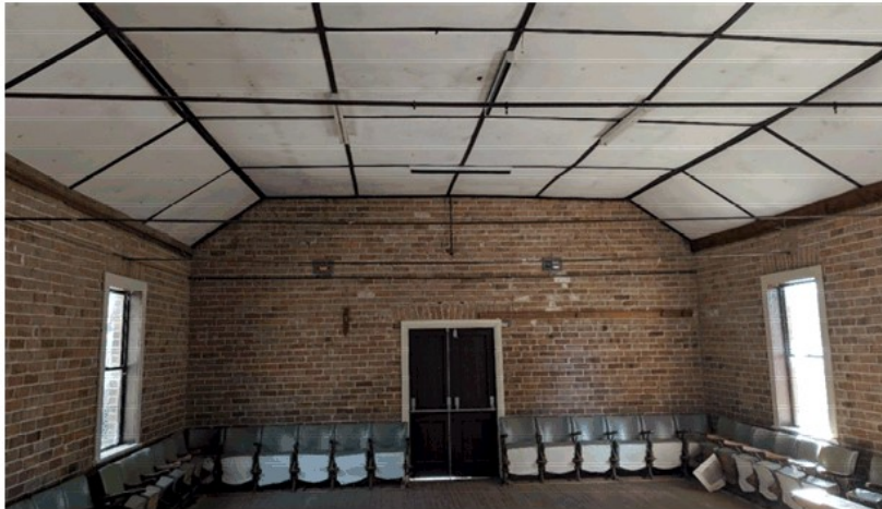
Figure 3 The structural tie rods need checking/confirming that they are sound. Review the centres of the lights with the electrician to ensure that the new pendants will be sufficient.
