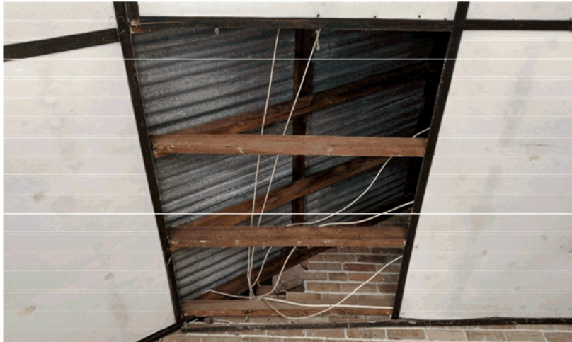
Figure 1 The timber framing appears sound from this view. Further exposure is recommended. Removal of the ceiling is acceptable given the value and importance in retaining the structure.
