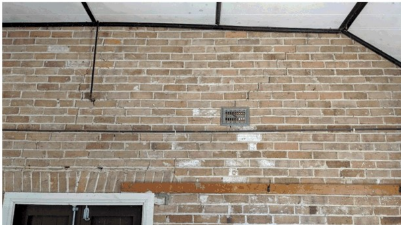
Figure 4 The end wall has the movement cracks plus the side wall. Both leaves of the brick will need to be stitched.
